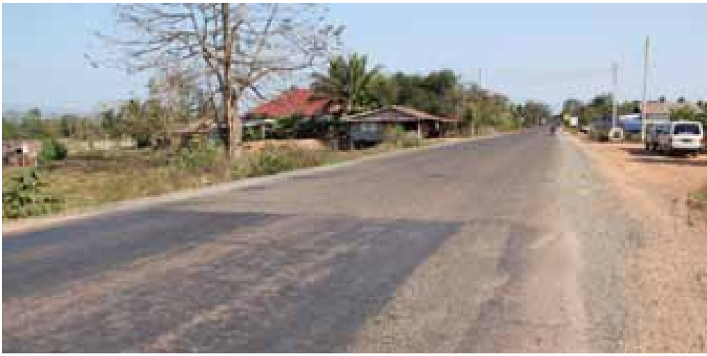
The connection between a road section repaired under the World Bank grant (bottom) and a section repaired using government funds (top) at Senxoom village in Phonhong district, Vientiane province.
